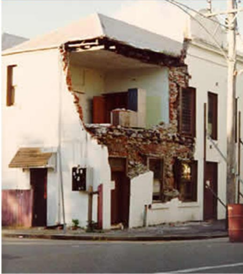
Hidden Treasure Hotel, Laman Street after the 1989 Newcastle Earthquake.
