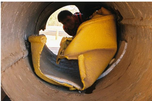
Earthquake damage in Western Australia. Main water supply pipe was telescoped by over one metre by the Meckering earthquake in 1968. Photo: Roz Kerr
